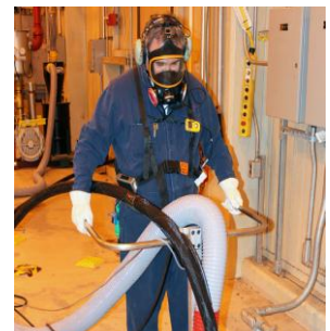
Mechanical Technician Tim Wilson lays out the Nitrocision system's scabble head in preparation for a training session. Systemization on the unit continues, but Wilson and the rest of the Nitrocision team are learning as much as they can so they'll be ready to begin hands-on training when the unit is operational.
