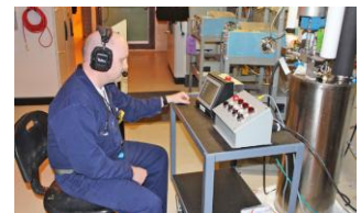
When the Nitrocision system is in use, ANCDF Instrument and Calibration Technician Jonathan Whiten will rely on the control panel, left, and backup control panel to monitor the metal tank in front of him, which is called the chiller.
